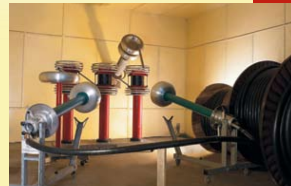
EHV Testing Facility
